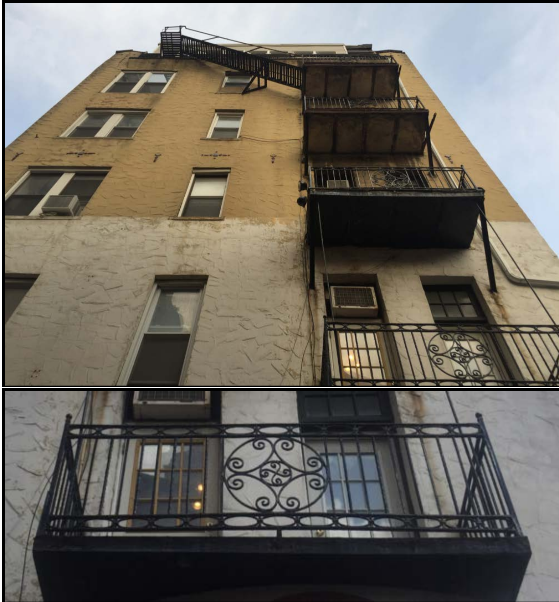
Top: Looking east at the upper floors of the S. Camac Street elevation, featuring wrought iron, Mission or Spanish-inspired balconies, and other discreet tile details. Bottom: A wrought iron balcony on the S. Camac Street elevation of the Camac Baths. Source: Oscar Beisert, 2018.
