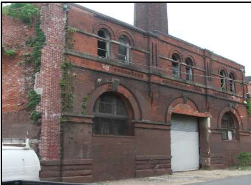
Weisbrod & Hess Brewery—Loading Room, Condenser & Storage (Building 1) and Boiler & Wash House (Building 2), 2117 E. York Street, Kensington, Philadelphia Nomination to the Philadelphia Register of Historic Places, Fall 2016 – Page 5
