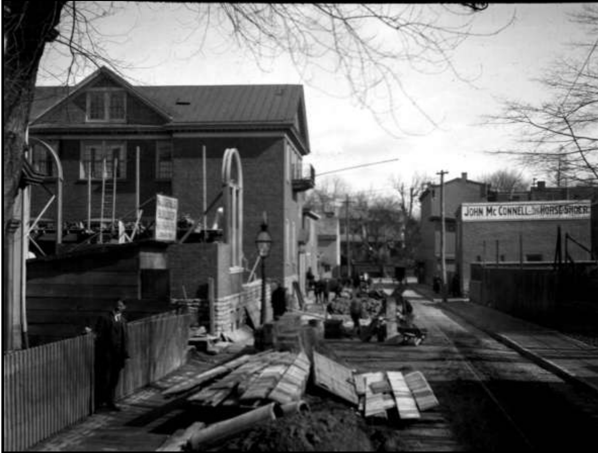
Looking at 25 and 27 W. Penn Street, this photo shows the construction of the 1908 Addition to the Germantown Boys' Club, designed by Mantle Fielding, Jr., ca. 1908. Photograph taken by Marriot Canby Morris. Courtesy the Library Company of Philadelphia.
