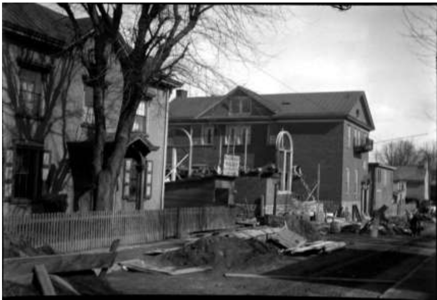
Looking at 25 and 27 W. Penn Street, this photo shows the construction of the 1908 Addition to the Germantown Boys’ Club, designed by Mantle Fielding, Jr., ca. 1908. Photograph taken by Marriot Canby Morris. Courtesy the Library Company of Philadelphia.
