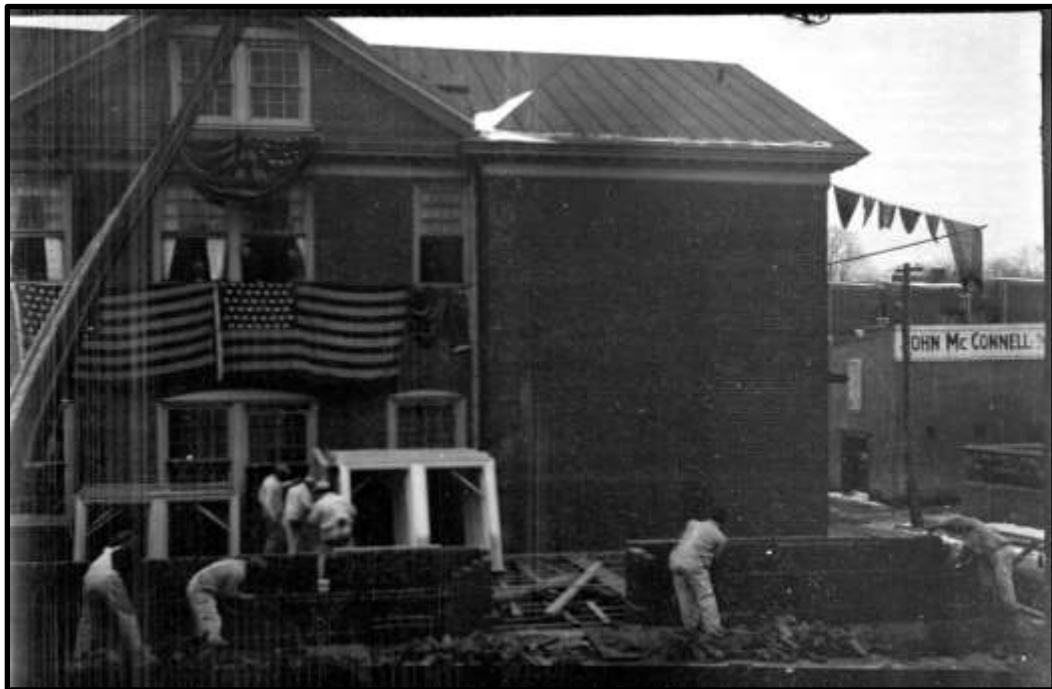
Photographs taken by Marriot Canby Morris of the construction of the 1908 Addition to the Germantown Boys' Club, ca. 1908. Courtesy the Library Company of Philadelphia.
