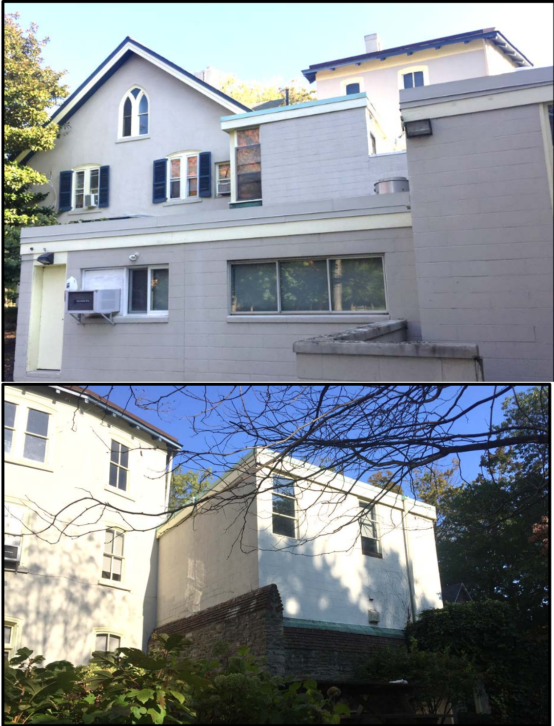
Figure 16. Top: The southwest elevation of the subject property with Addition 1 in the foreground. Bottom: The rear elevation of the subject property, Addition 3 is the two-story block building in the foreground at center and is considered non-contributing. The three-story building of left and the stone wall beneath the Addition 3 are both contributing. Source: Oscar Beisert, 2018.
