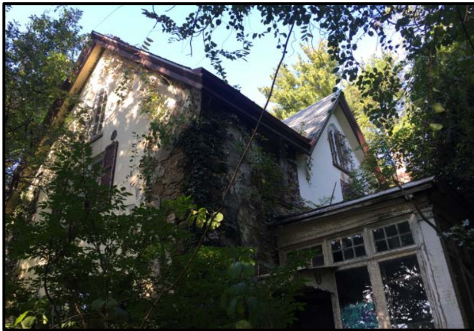
Figure 21. The southeast and rear (northeast) elevations of the cottage, stable, or residence and carriage house-stable building that was formerly associated with the subject property. Source: Oscar Beisert, 2018.
