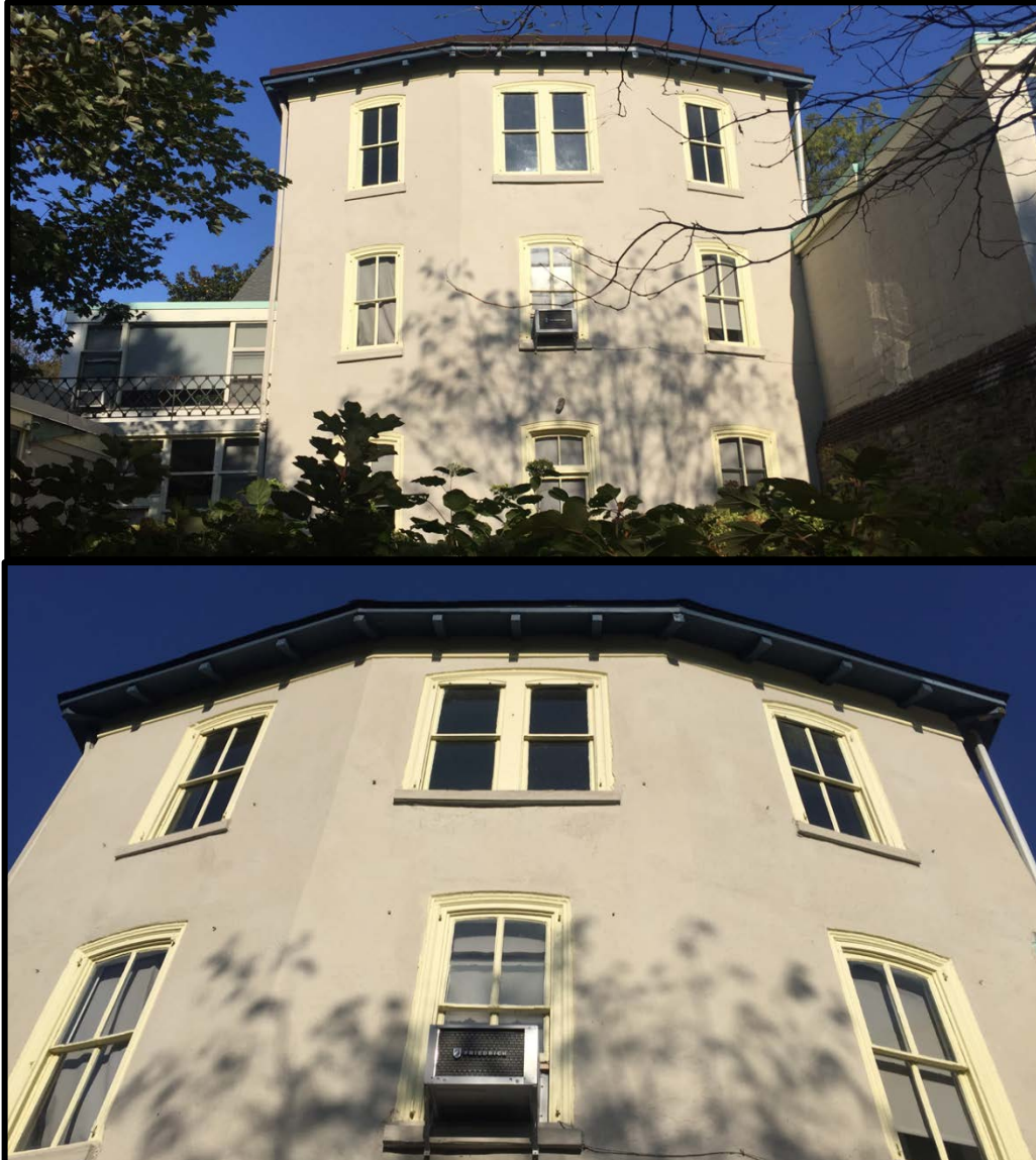
Figure 9. Top: The rear (southeast) elevation of the subject property. Note that the three-part façade features windows at each floor that are almost entirely original and/or early two-over-two wooden sash configuration. Bottom: The upper two floors of the rear (southeast) elevation. Source: Oscar Beisert, 2018.
