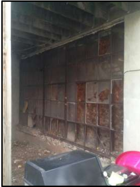
Looking northwest at a multi-light industrial metal window within the stable. Courtesy Oscar Beisert.
