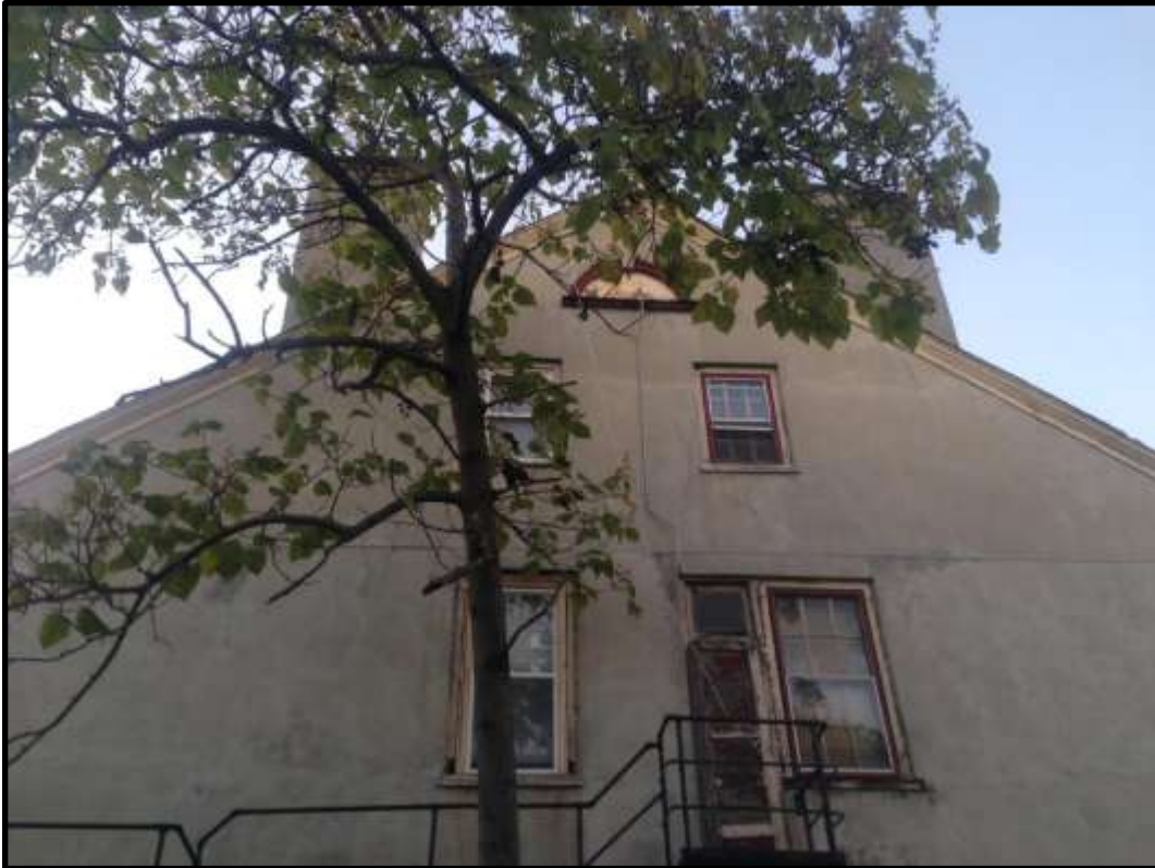
Looking northwest at the upper floor and gable of the southeast facing elevation. Courtesy Oscar Beisert.
