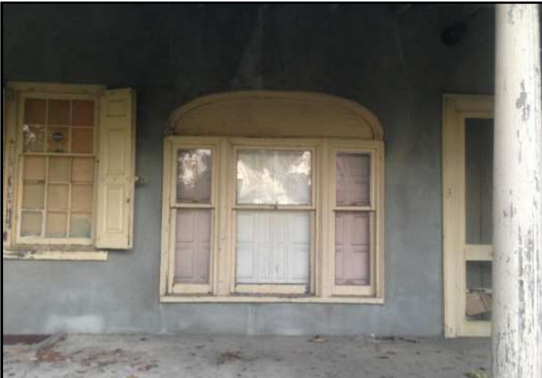
Looking southwest within the porch of the rear elevation. Courtesy Oscar Beisert.
