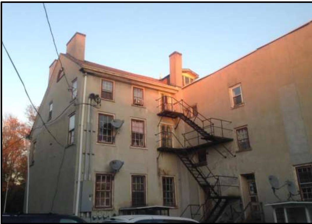
Looking northeast, note that the rear elevation of the building is a full three stories with many original and/or older wooden sash windows. A single dormer pierces the rear roof. Courtesy Oscar Beisert.
