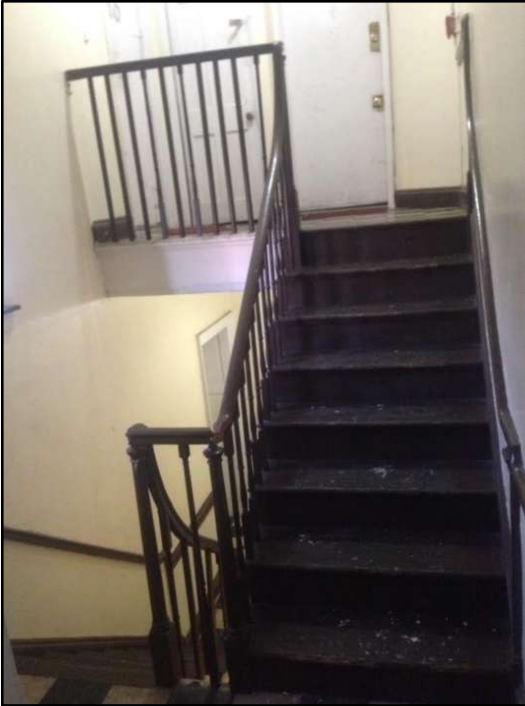
Standing on the landing between the second and third floors, many original details exist. Courtesy Oscar Beisert.
