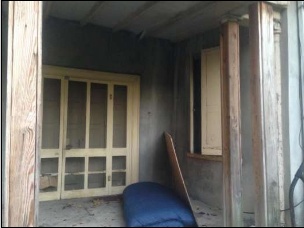
Looking northwest within the porch of the rear el. Courtesy Oscar Beisert.
