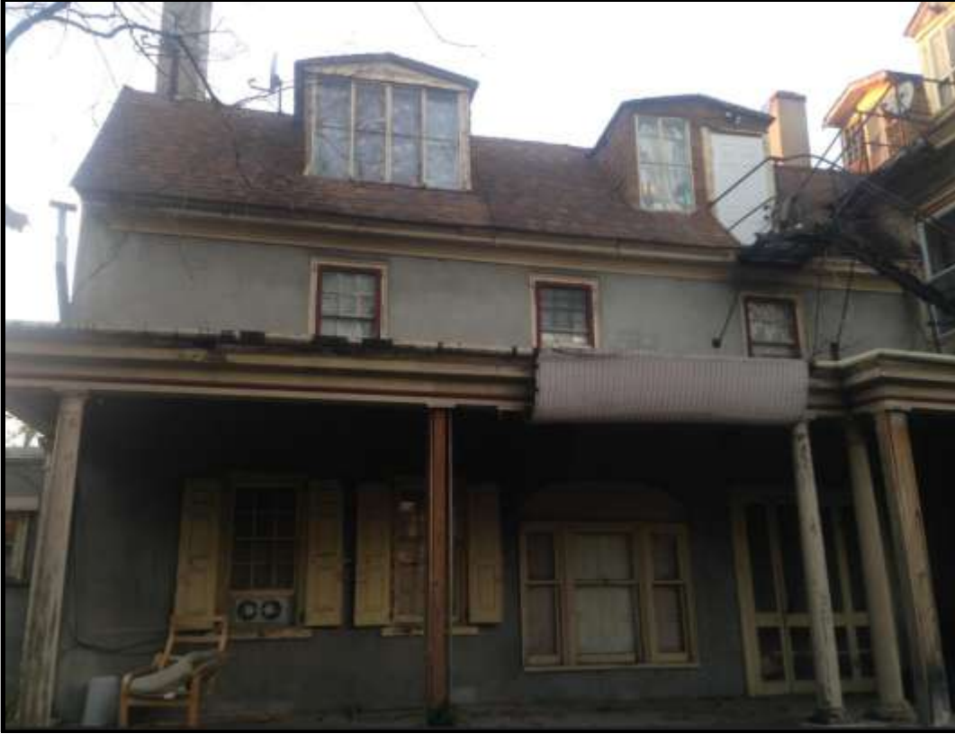
Looking northwest at the massive rear elevation and its porch. Note many of the features at this elevation have been replaced. Courtesy Oscar Beisert.
