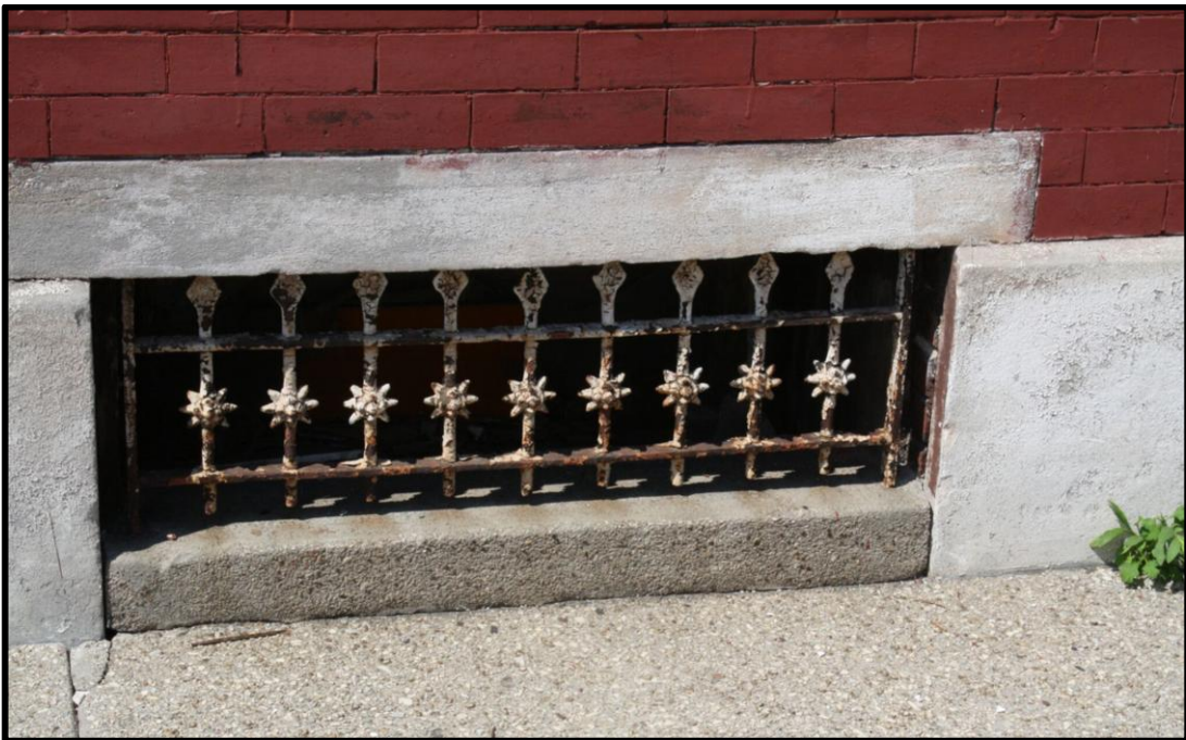
Looking north. Likely original, the basement windows are shielded by ornamental cast iron grills. Courtesy Janette Amstutz.
