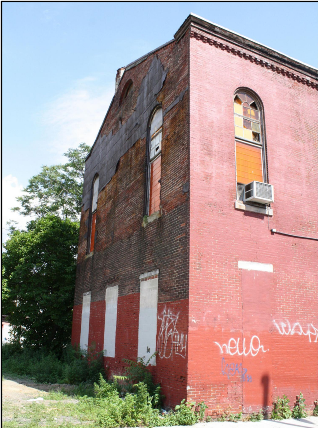
Looking southeast. The rear elevation features two arch-topped windows in the second floor and three rectangular openings that are shuttered. Courtesy Janette Amstutz.
