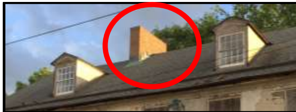
The chimney of the subject house at 5112–14 Germantown Avenue. Courtesy Oscar Beisert.
