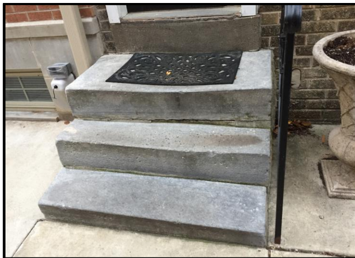
Looking east, the original marble steps of the subject house. Source: Oscar Beisert.
