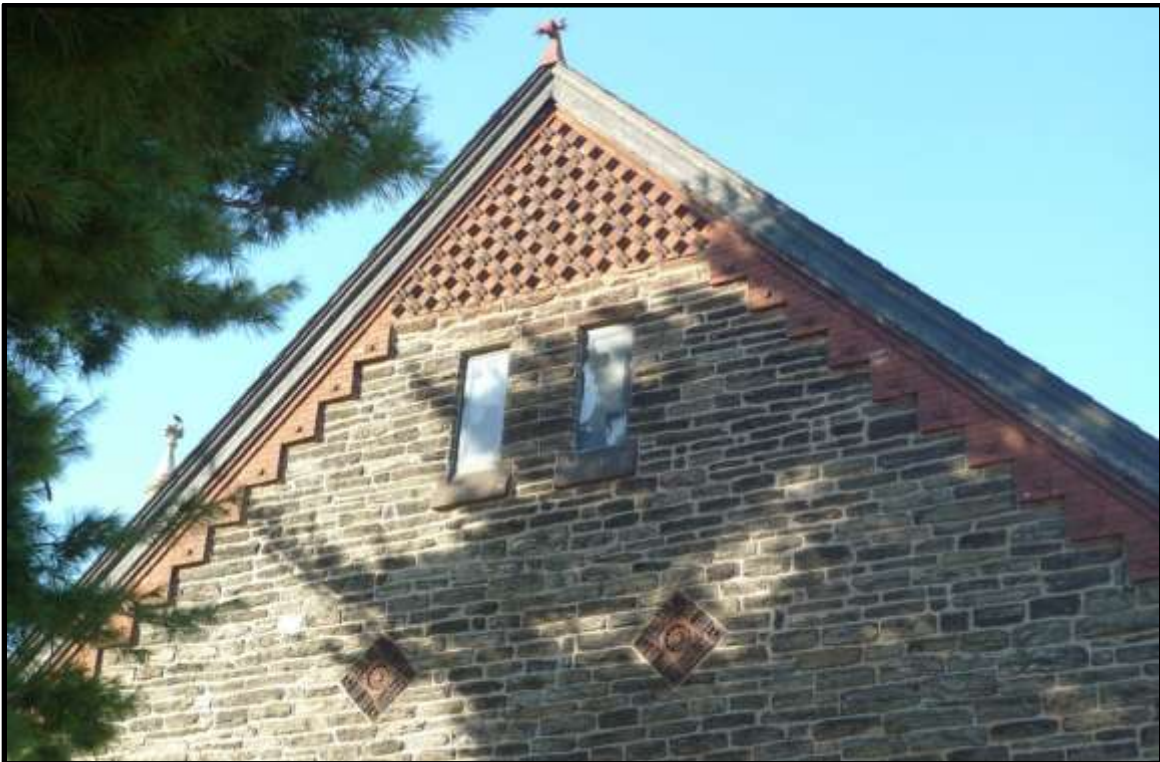
Detail at the southwest gable of the Sunday School showing decorative brickwork. Source: J.M. Duffin.
