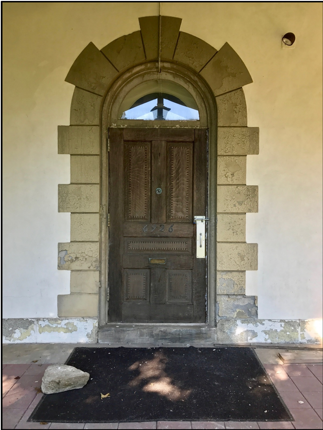
Looking west at the Primary Entrance within the Primary Elevation. Source: Brad Maule.
