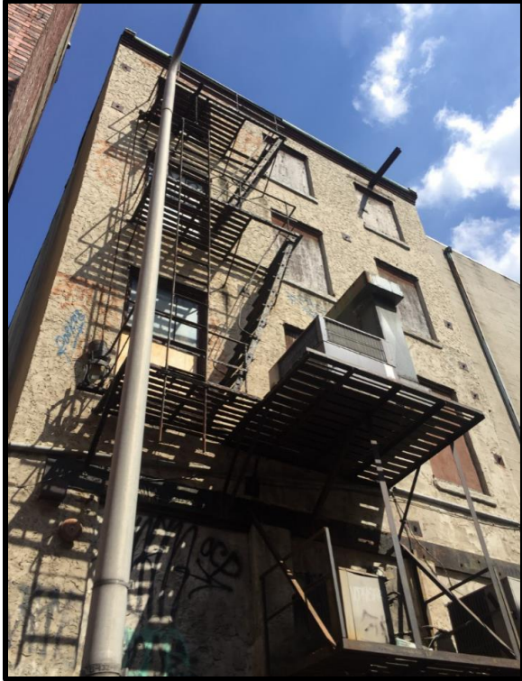
Figure 9: The rear (south) elevation along Ionic Street, which was the manufactory and warehouse. Source: Oscar Beisert, 2018.
