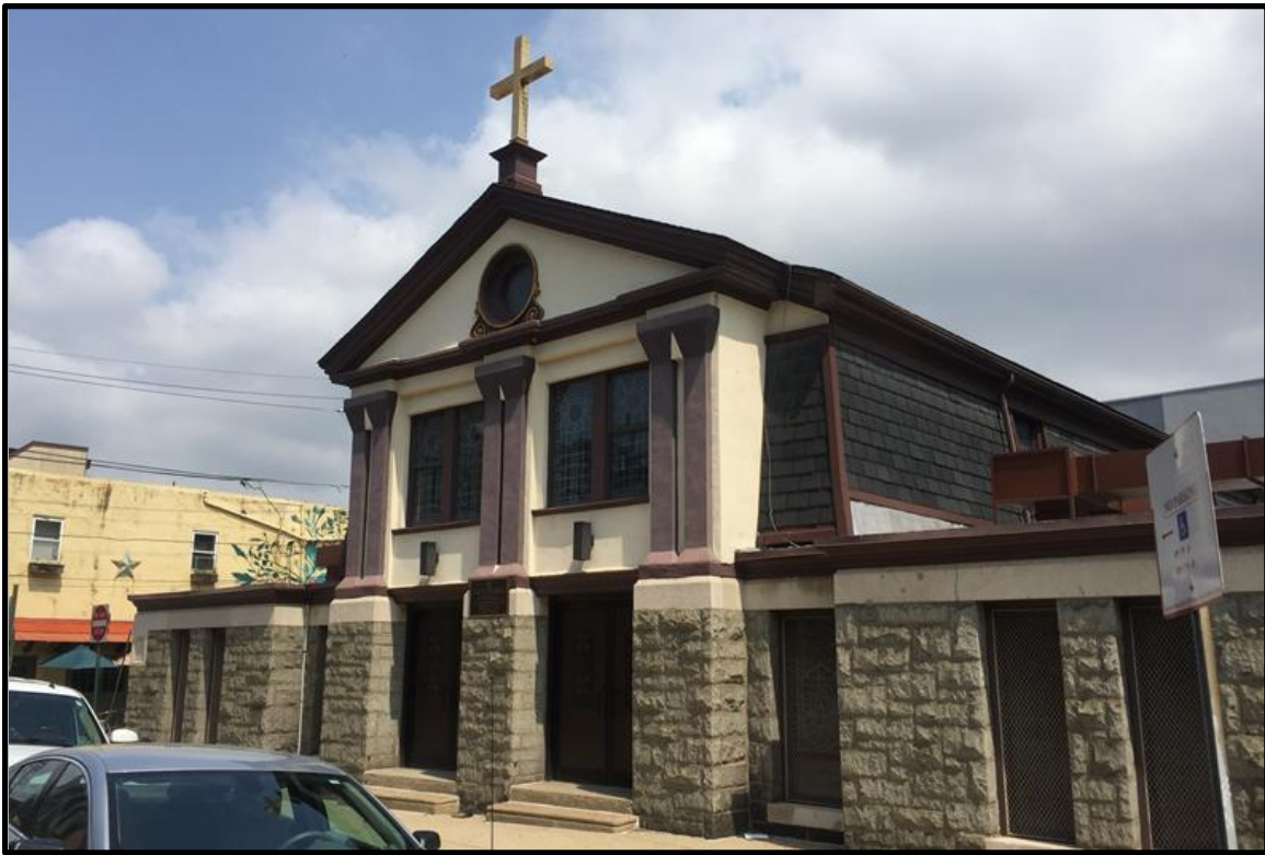
Looking northwest at the church of St. Agnes, showing the gambrel roof that is obscured by the central façade. Source: Oscar Beisert.
