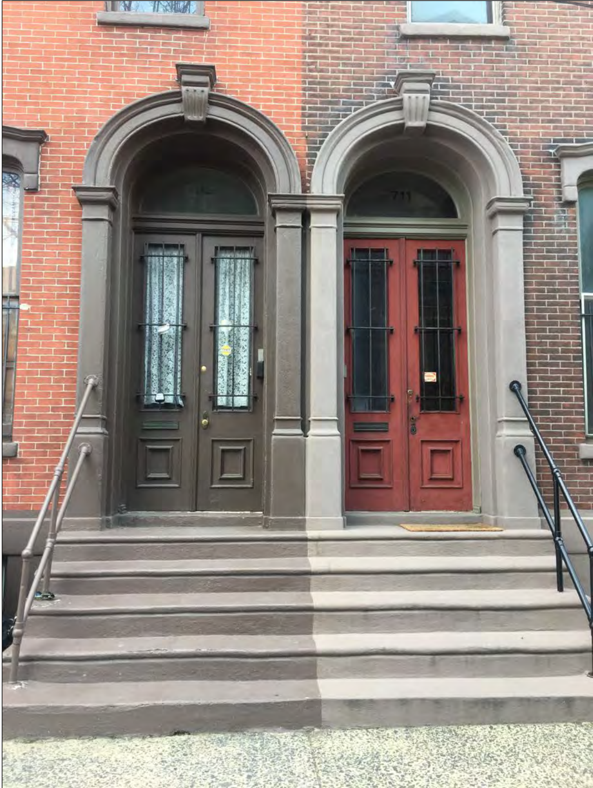
Figure 7. Shared steps leading to doorways of 711-713 N. 6 th Street. 713 N. 6 th Street is to the left. Photo taken by Arielle Harris, April 2018.
