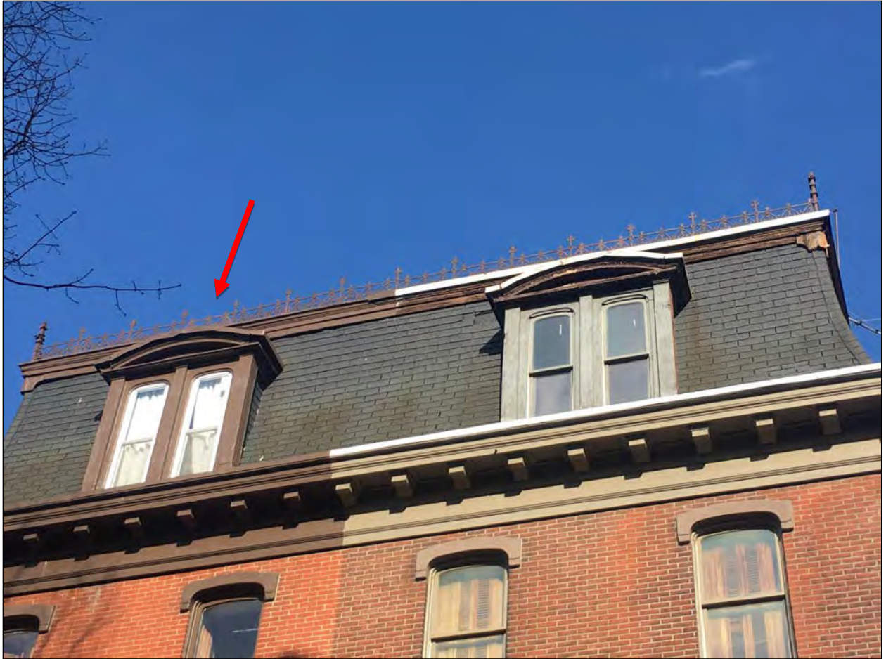
Figure 11. Detail of cornice and cast iron cresting at 711-713 N. 6 th Street. Photo taken by Arielle Harris, April 2018.
