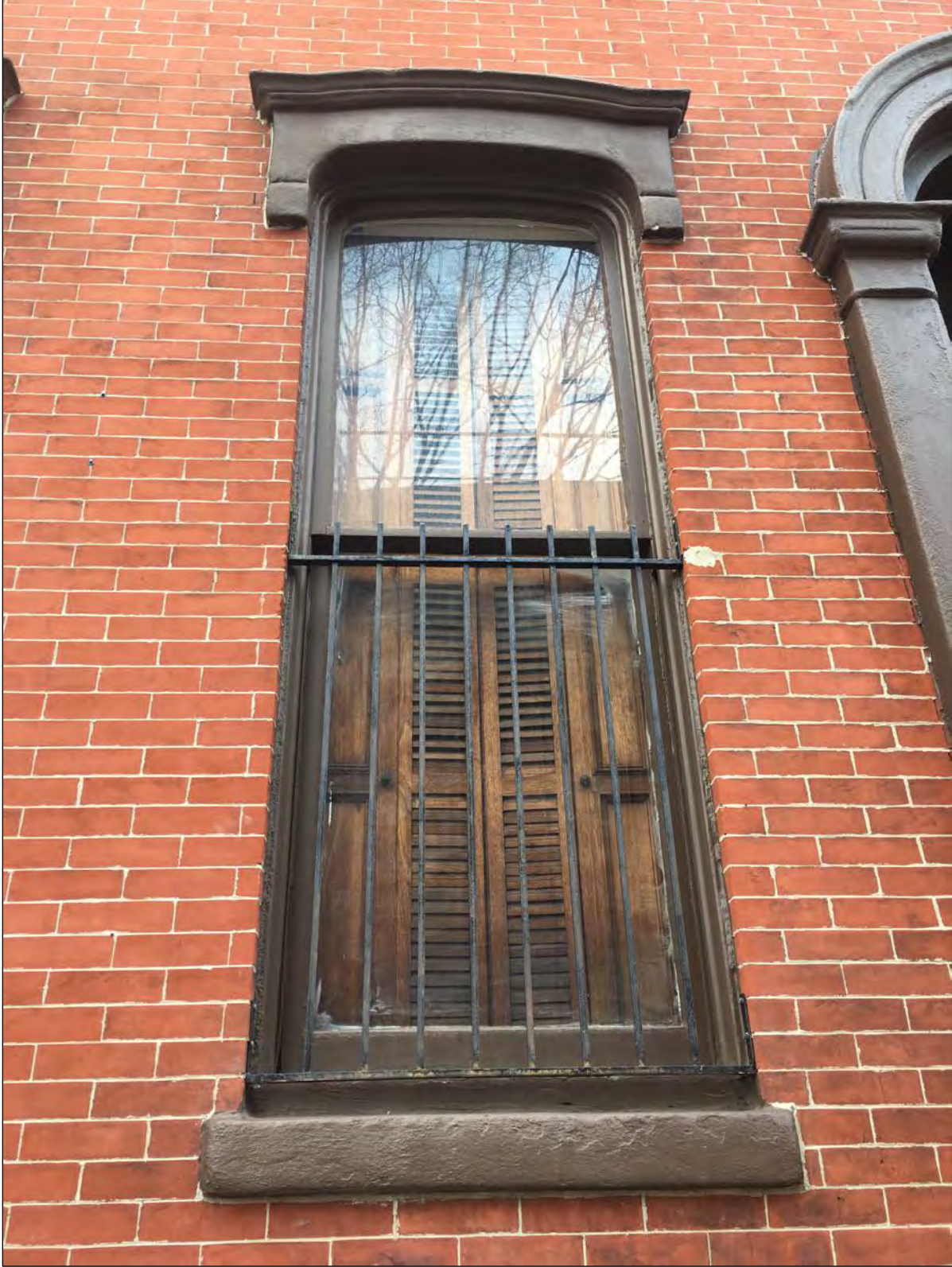
Figure 9. Detail of first floor window at 713 N. 6 th Street. Marble sills and lintels have been painted brown. Original folding door shutters can be seen within. Photo taken by Arielle Harris, April 2018.
