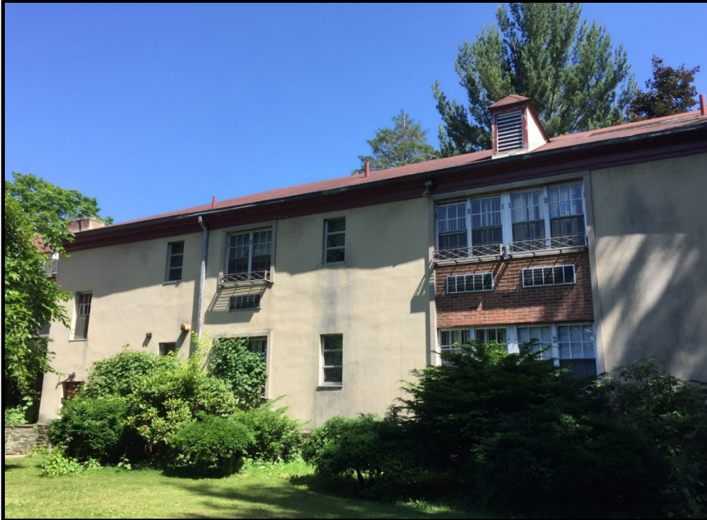
Photo No. 35: Looking east at the rear elevation of the institutional addition (post-1945). Source: Keeping Philadelphia, 2018.
