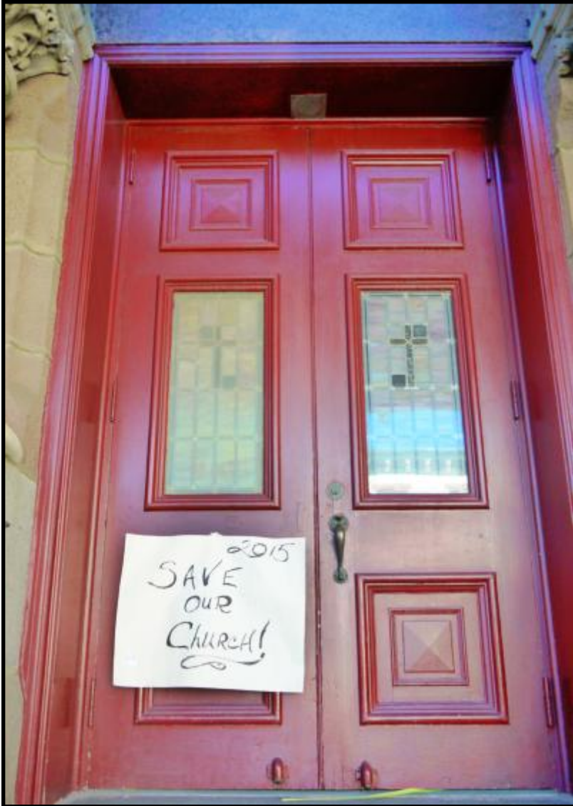
Looking southwest, the original central doorway and its original and/or period-appearing doors.
